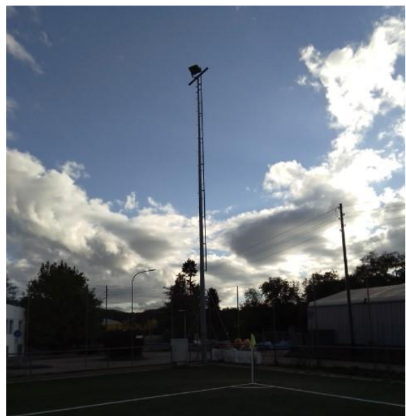
Luminaire B8 – Terrain B
